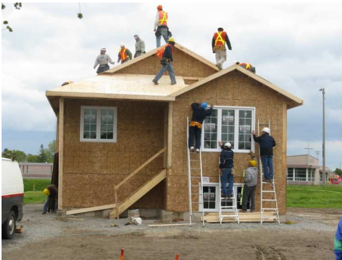
On that day, 70 volunteers framed and sheathed the walls, installed and sheathed the trusses and installed the exterior doors and windows. Construction began at 9:30 AM and concluded by 2:15 PM.
